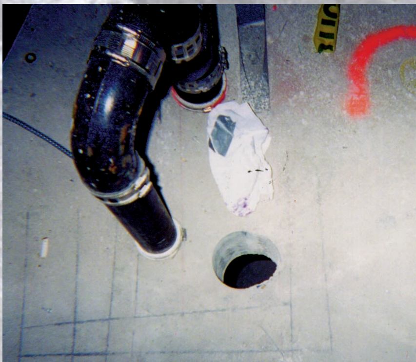
The mechanical contractor is able to drill the hole by staying away from marks which represent cables.
